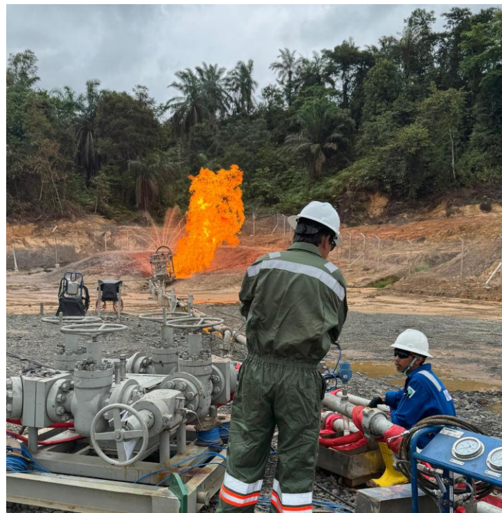
SEM-01 Well Test – August 2025
